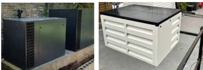
Figure 8: Some example of extra acoustic casing for the heat pumps.
